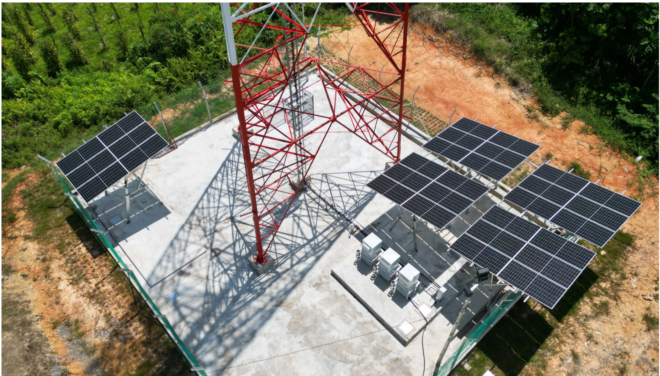
Huawei helps REDtone build green sites in Malaysia
