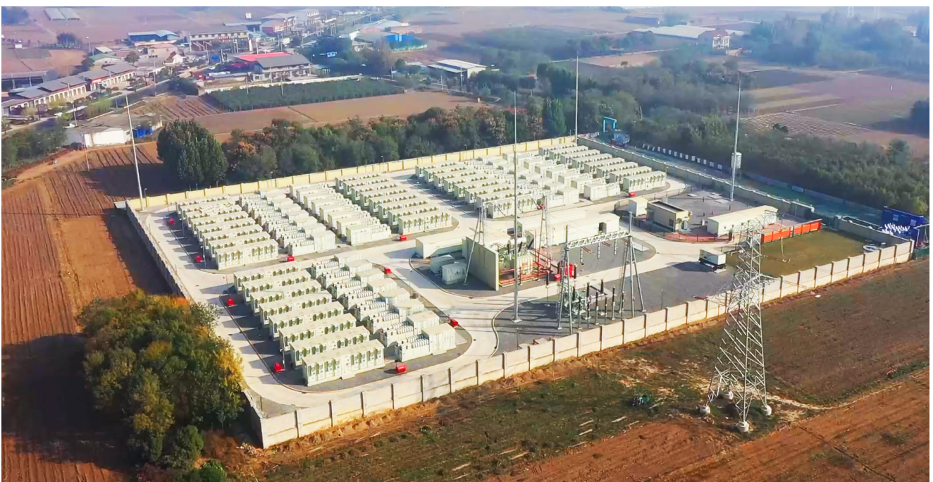
Huawei helps the largest energy storage plant in Neihuang County generate power
