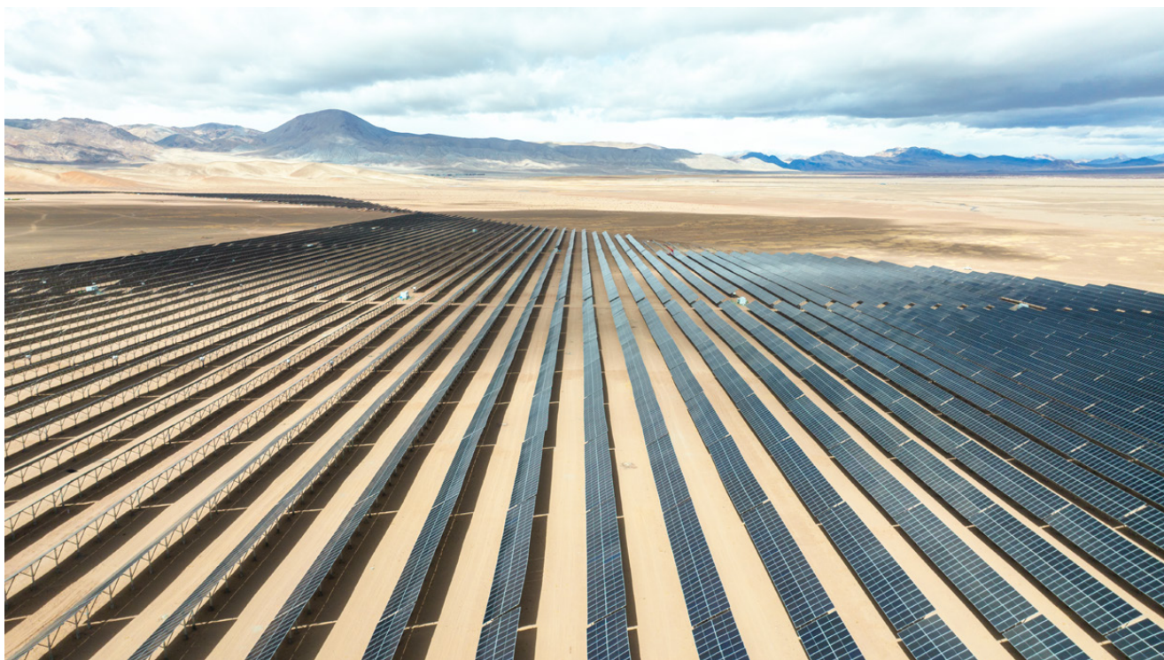
Zero-carbon PV + ESS + Heating demonstration project in the Ngari Prefecture developed by CGN and Huawei
