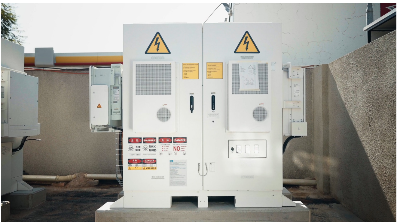
Huawei's ESS helps a commercial building in South Africa generate clean power
